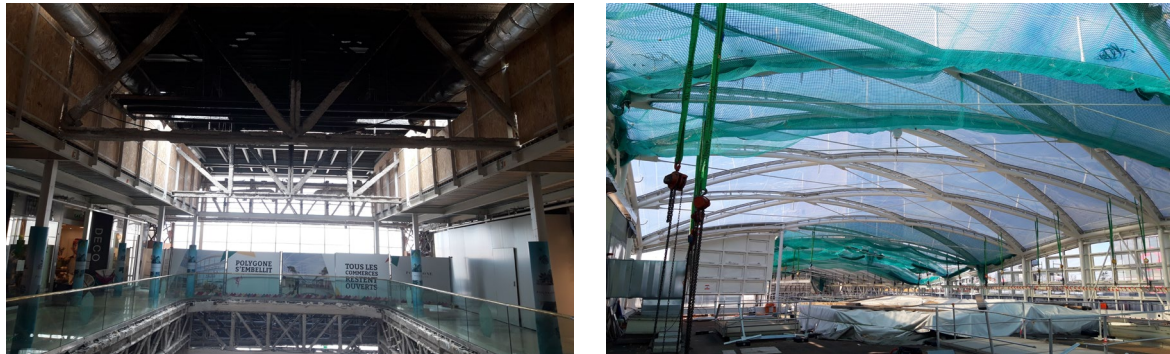
Figure 3: On the left, the shopping centre remains open during the renovation work; on the right, the ETFE cushion roof is being installed over the existing roof.
