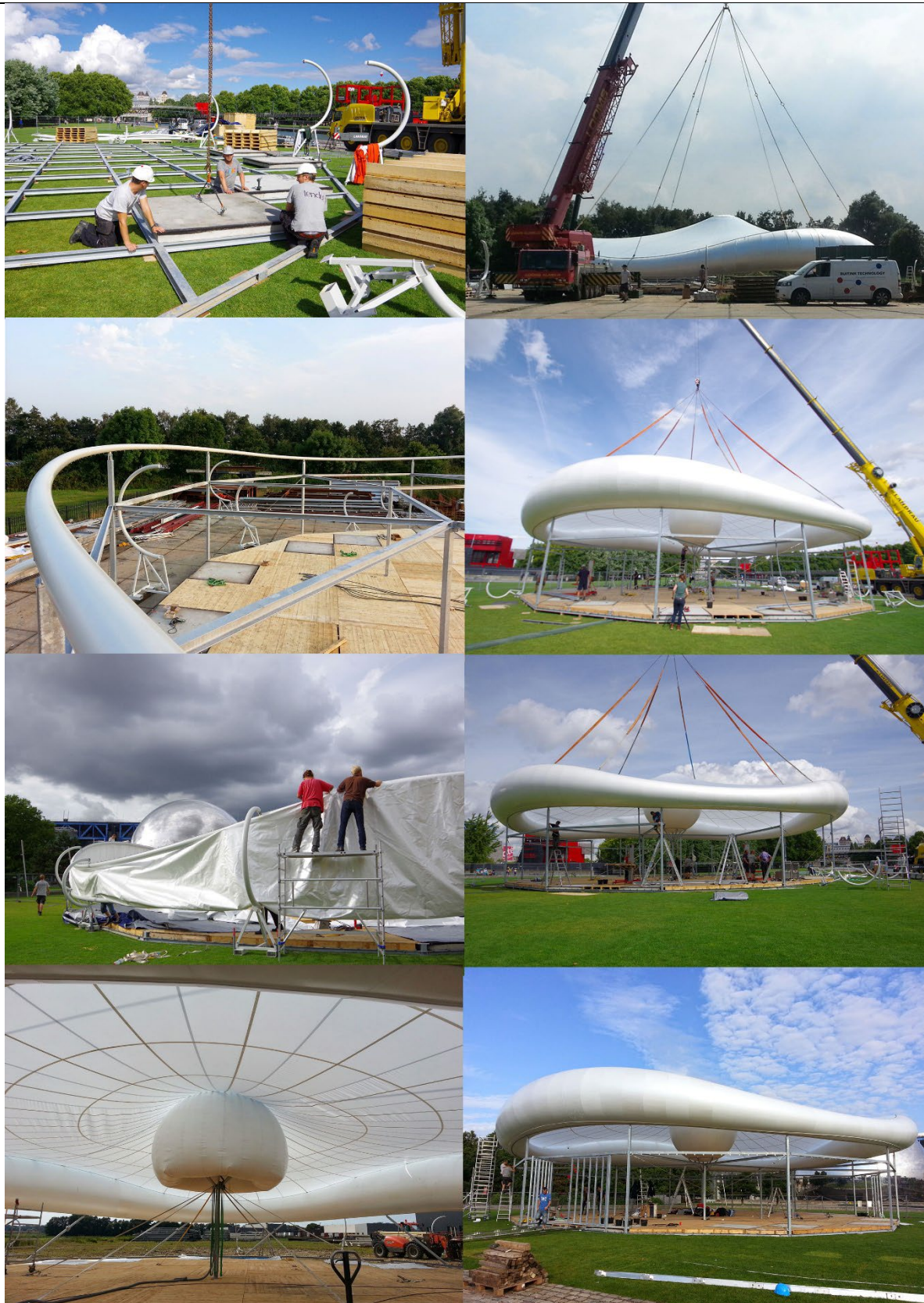
Figure 8: installation of Wave Pavilion structural floor & roof lifted by a crane for supporting structure installation
